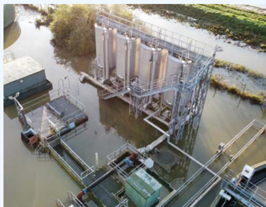
Anwick Water Recycling Centre under water. Image credit: Paul Barham, Maintenance Support Technician.
